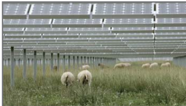
Farm solar generation system
